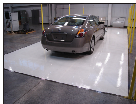
RapidShield™ Quality Inspection Area
