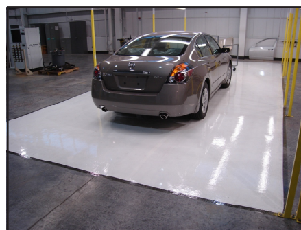
RapidShield™ Quality Inspection Area
